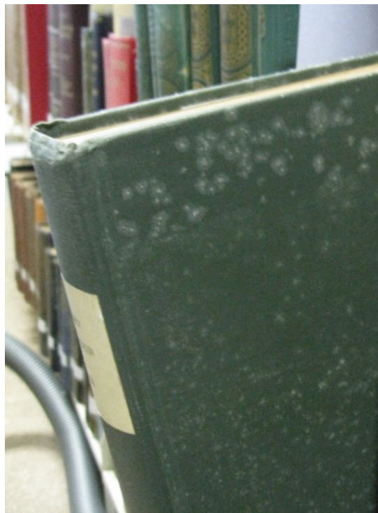
Mold outbreak caused by HVAC malfunction
